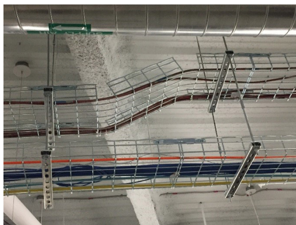
Figure 1: Wire mesh trays showing separation of power and data cables in an office building.
